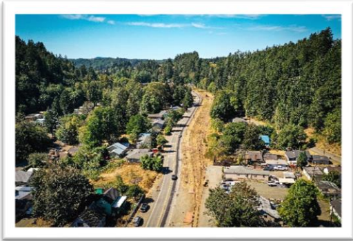
Western Gateway project begins on West Railroad Avenue from Pacific Court through 8 th Street
